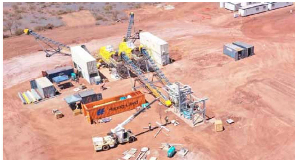
Stage 1 construction of the Butcherbird manganese project is on track to be completed this month
